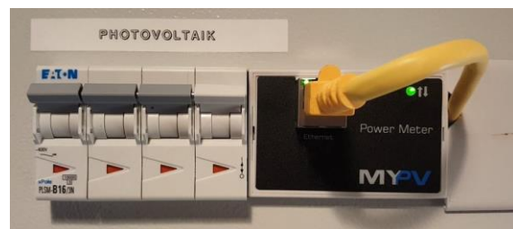
Figure 3: The my-PV Power Meter is mounted in the distribution cabinet directly after the utility meter.
