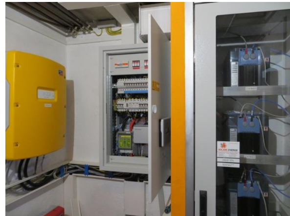
Figure 1: SMA Sunny Island (left) and battery packs (right)
