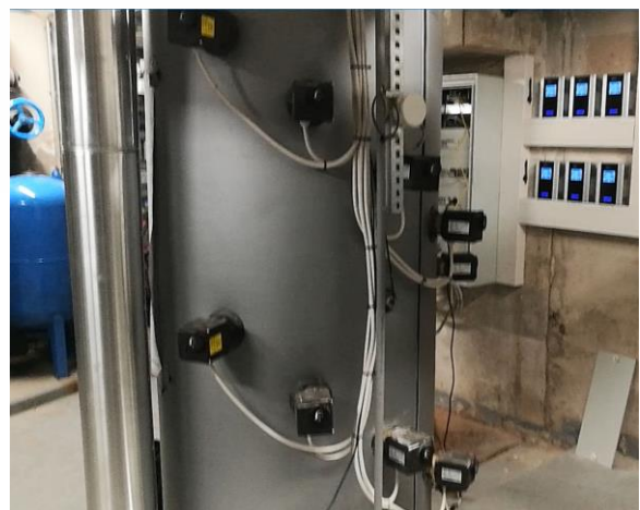
Figure 2: Storage tank with my-PV immersion heaters
