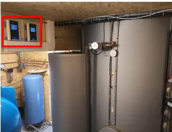
Figure 2: AC•THORs for hot-water preparation
