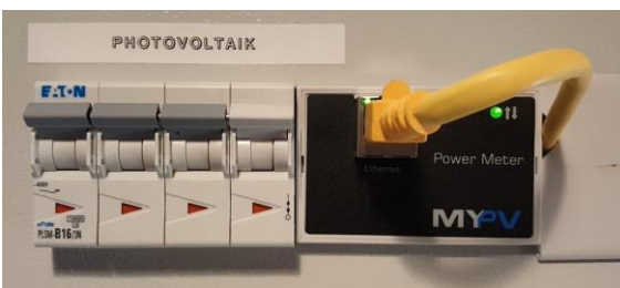
Figure: The my-PV Power Meter is mounted in the distribution cabinet directly after the utility meter.
